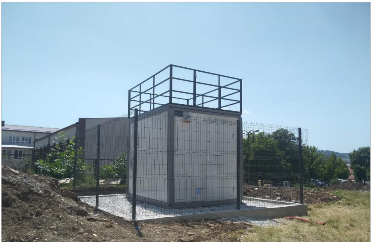
Photo 6- Custom made technical equipment container with handrails on the roof
